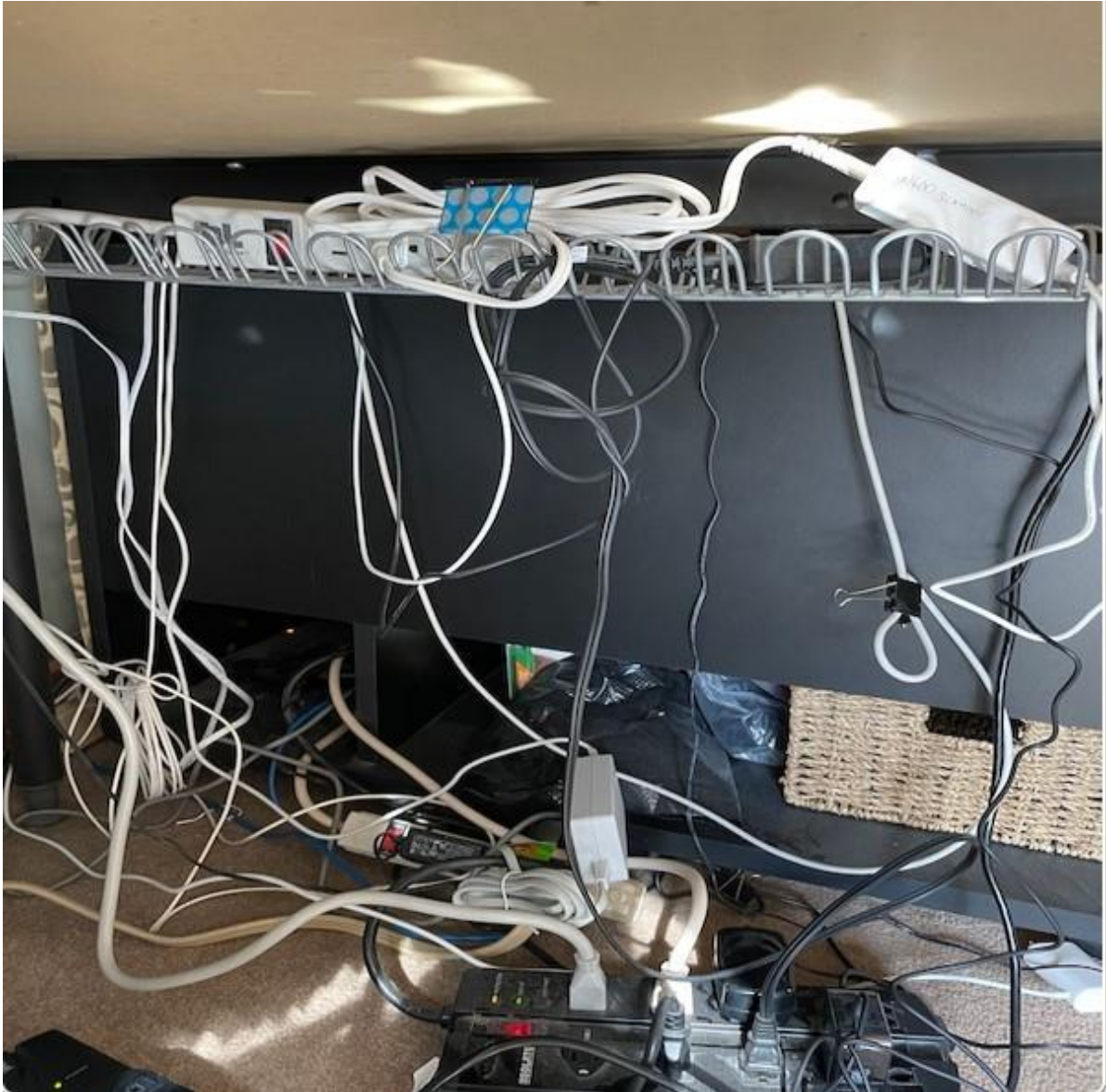
The room was a mass of cables; the cable to human ratio was almost disconcerting.
